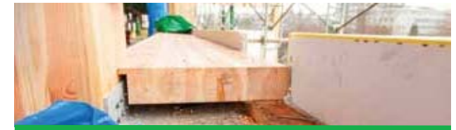
A section of the perimeter beam that resists the horizontal forces on the external wall of the building Photo: KK Law, Courtesy: naturally:wood
