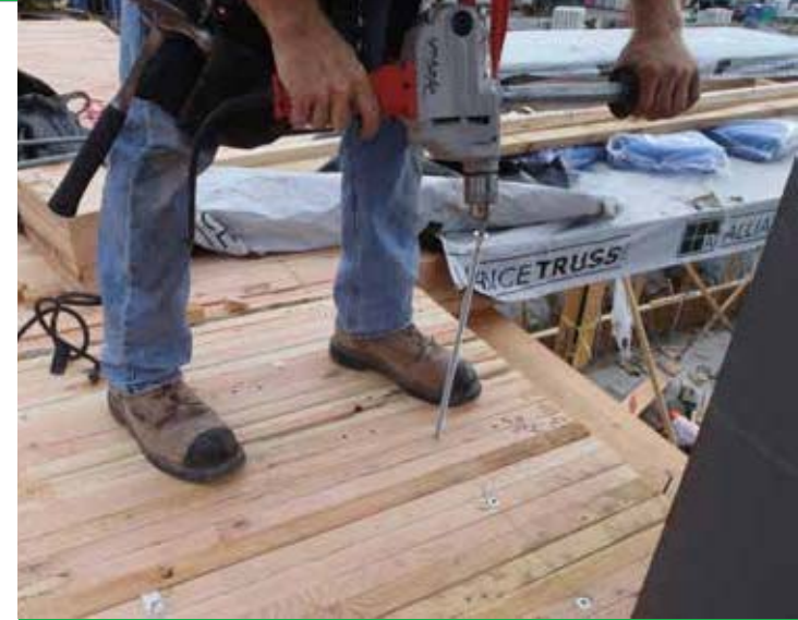
Once in place, the floor panels were lag screwed into the glulam beams Courtesy: Proscenium Architecture
