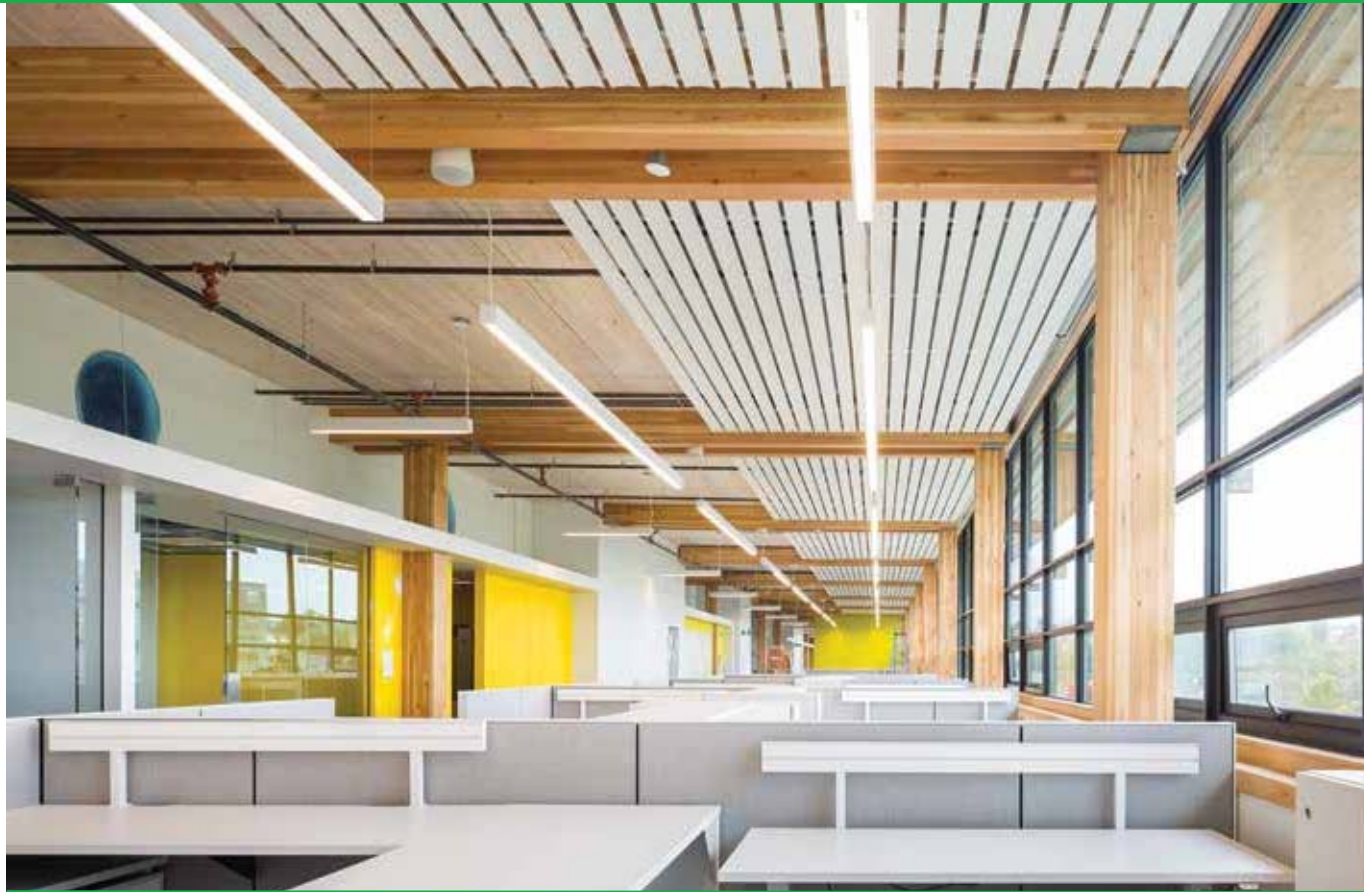
Radiant ceiling panels are positioned alongside the windows to provide additional heating or cooling as required Ed White Photographics
