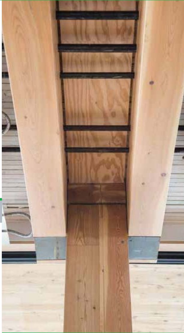
Connection between paired beams and column viewed from below Photo: KK Law, Courtesy: naturally:wood
