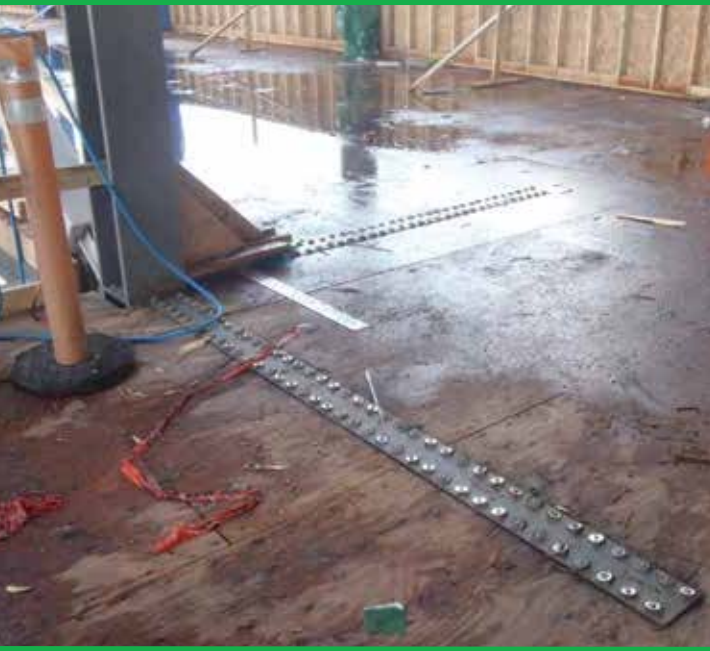
Steel strap tying wood floor to steel frame for lateral bracing Courtesy: Fast + Epp
