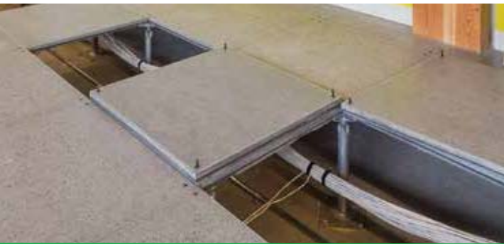
Access flooring. For a building of this size and type, the concealed space must be non-combustible.
