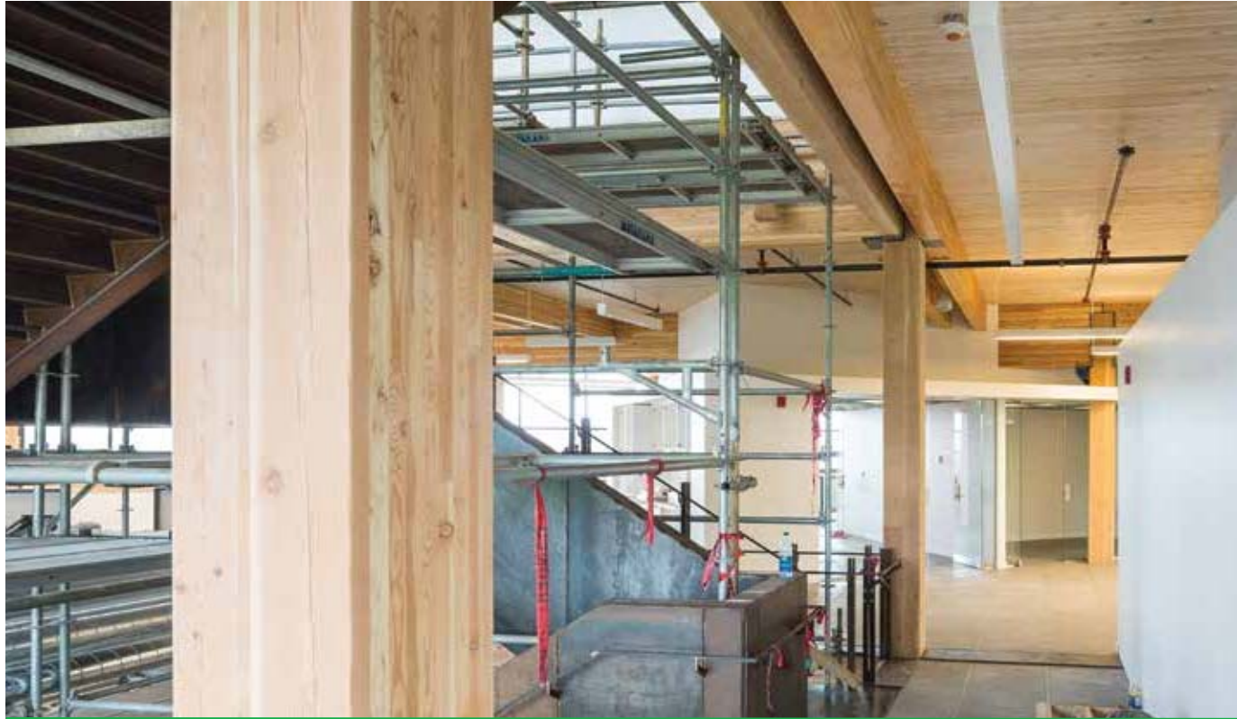
The dropped beams around the perimeter of the atrium are designed to contain smoke in the case of a fire
