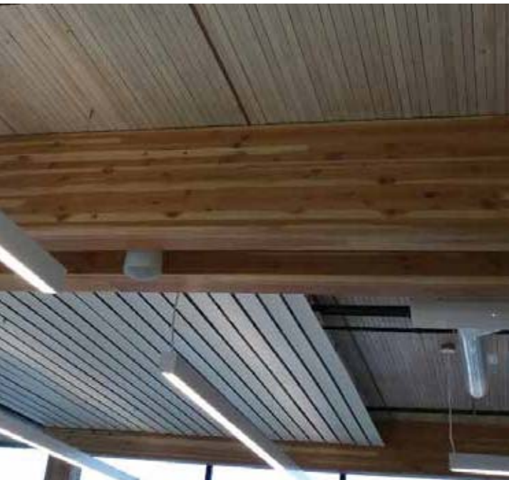
Small gaps were filled with mineral wool insulation and sealed with fire-rated caulking to meet fire separation requirements. Oversize gaps also had wood filler strips nailed in place from below. Courtesy: Ventana Construction
