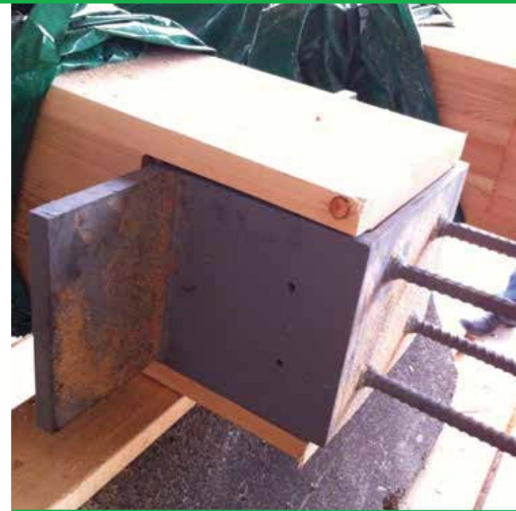
The columns have end-to-end bearing to minimize shrinkage over the height of the structure. Rebar rods on the saddle connector fit into holes drilled in the base of the column above. Courtesy: Fast + Epp
