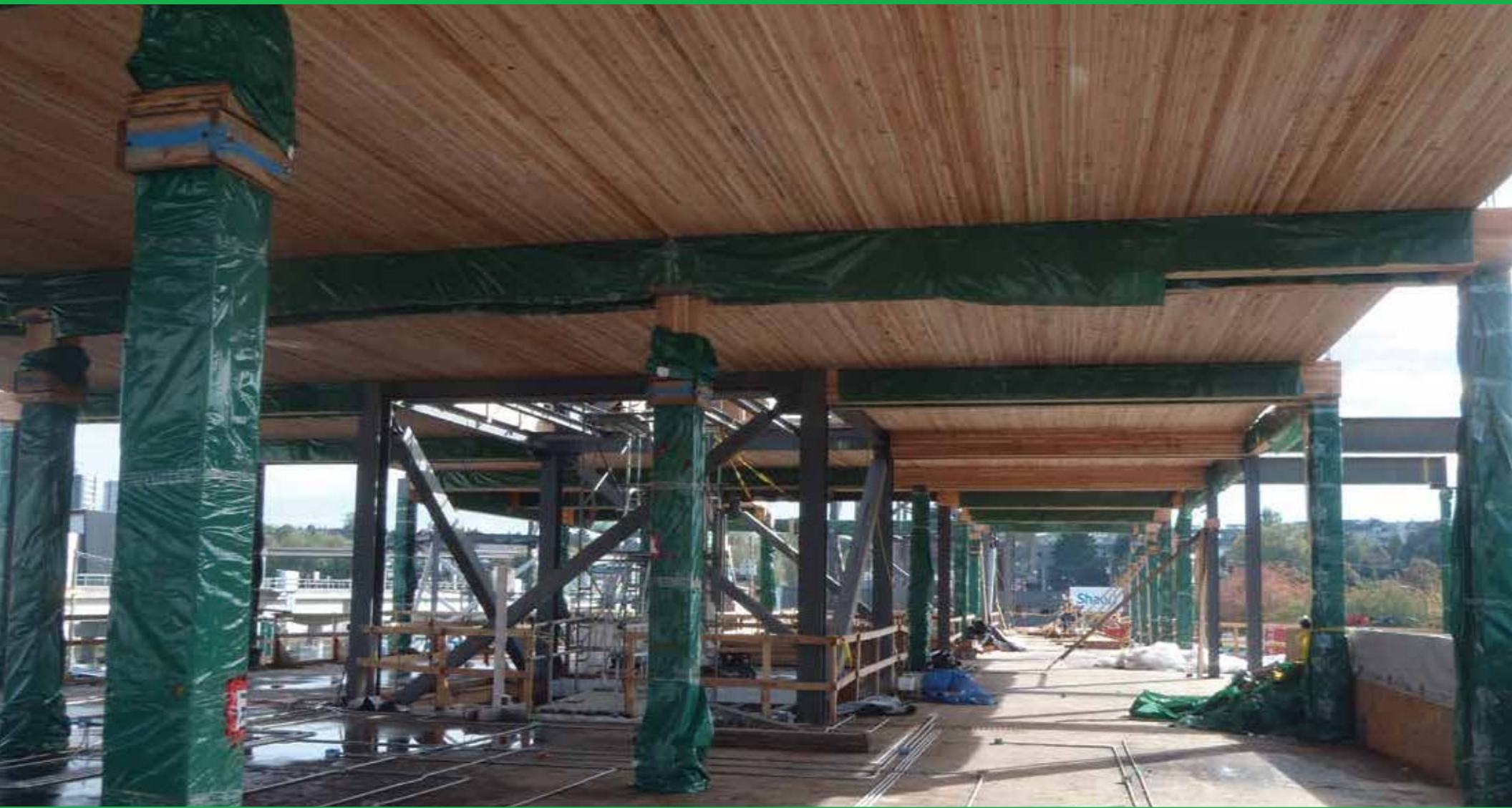
The nail-laminated floors are tied into braced steel frames that provide lateral resistance to the structure Courtesy: Fast + Epp
