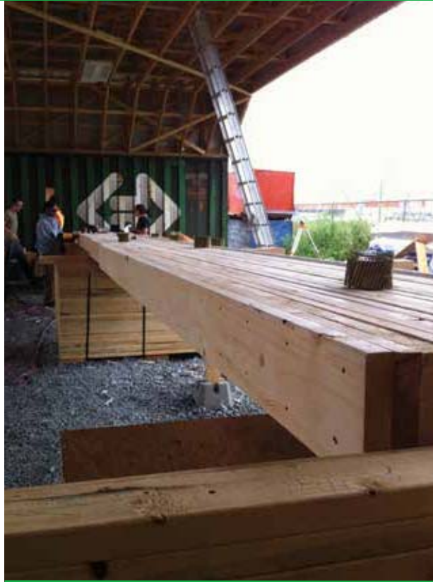
The floor construction resembles that of late 19th and early 20th century commercial buildings across Canada. This technique is being revived and updated to reduce the environmental impact of new buildings. Courtesy: Fast + Epp
